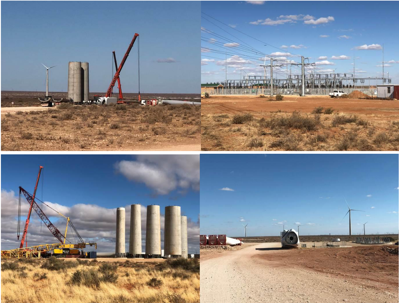
Figure 2-4: Photographs depicting the construction phase of a wind farm similar to De Rust South WEF.
