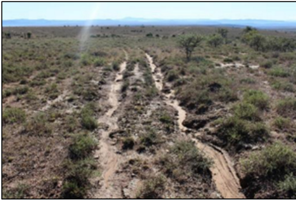
Figure 2.13. Lack of water runoff management on the Eskom Service roads
