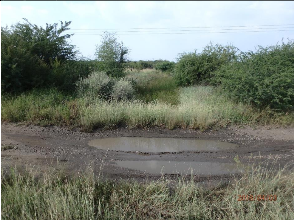
Drainage line filled with aquatic vegetation immediately adjacent the railroad at culvert No. 1 (on Figure 4.10). GPS coordinates: 32°48'7.48"S, 26°46'47.90"E.
