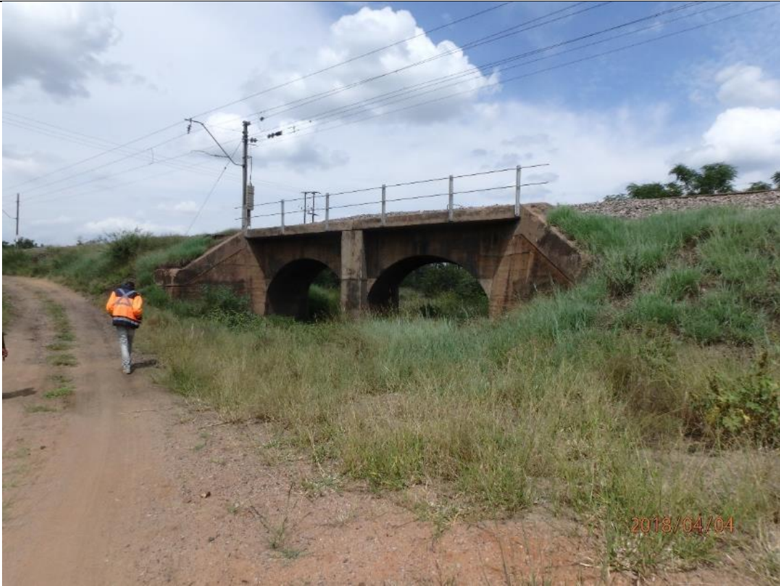
The rail bridge over the existing river near the Glencore smelter end of the project area (No 6 on Figure 4.10). GPS coordinates: 25°29'52.24"S, 27° 6'13.52"E.
