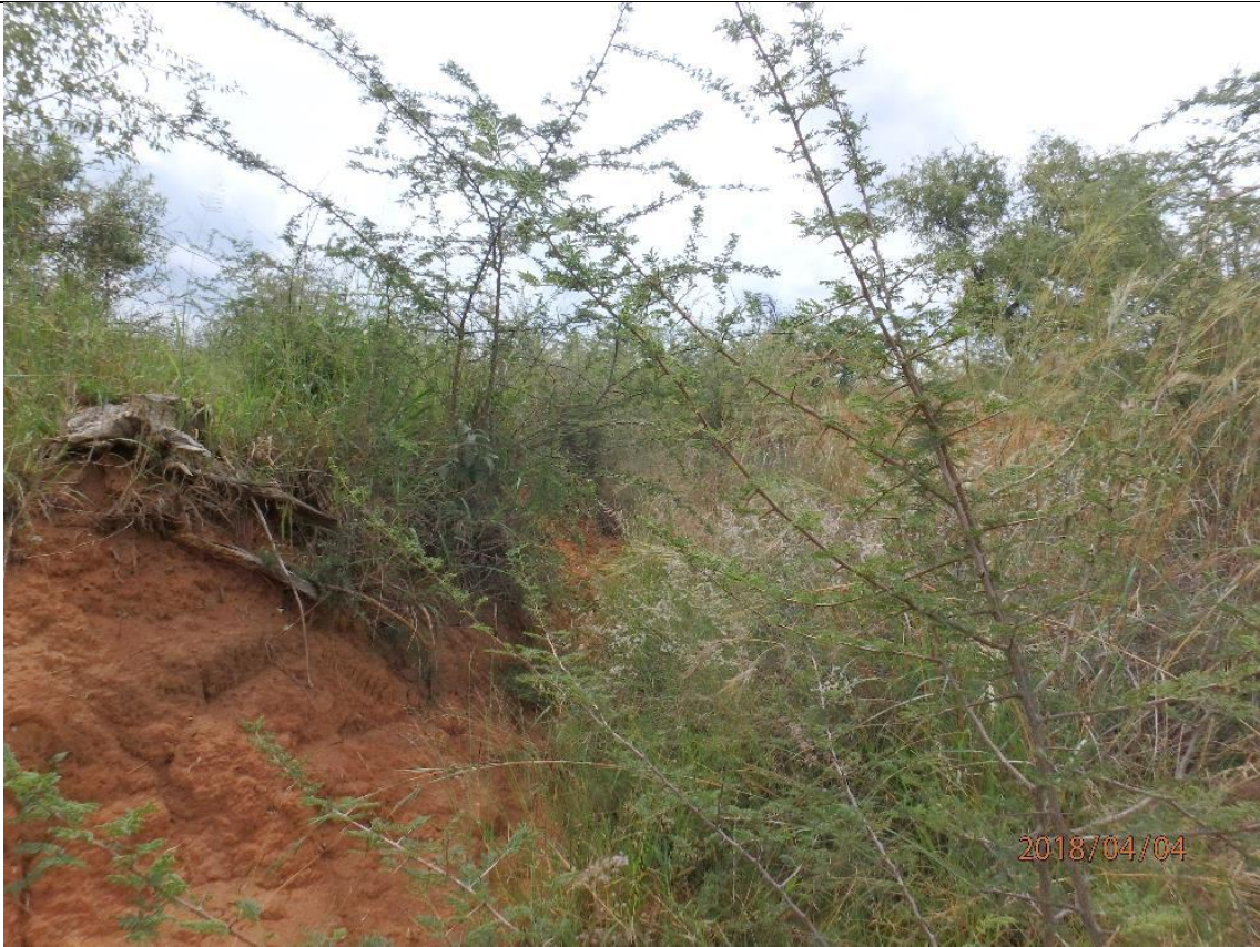
Drainage line filled with terrestrial vegetation immediately adjacent the railroad at culvert No. 4 (on Figure 4.10). GPS coordinates: 25°30'5.46"S, 27° 6'35.39"E.
