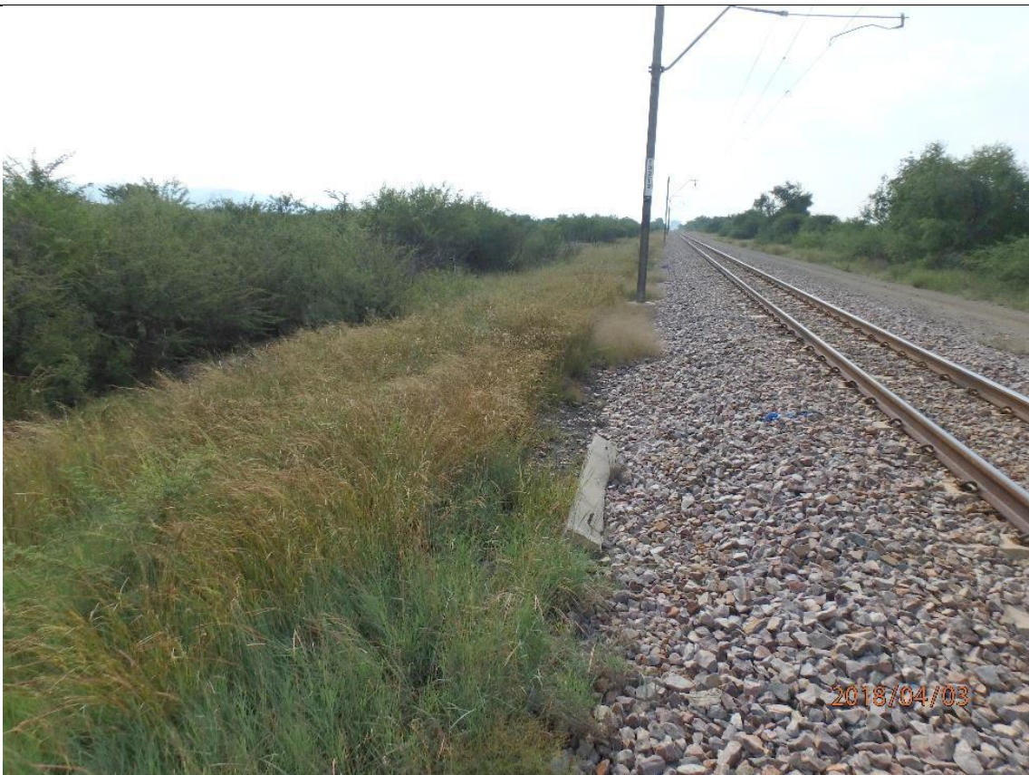
General view of the railway verge on the side without the access road (i.e. southern facing side). Note the rock verge used to stabilise the tracks.
