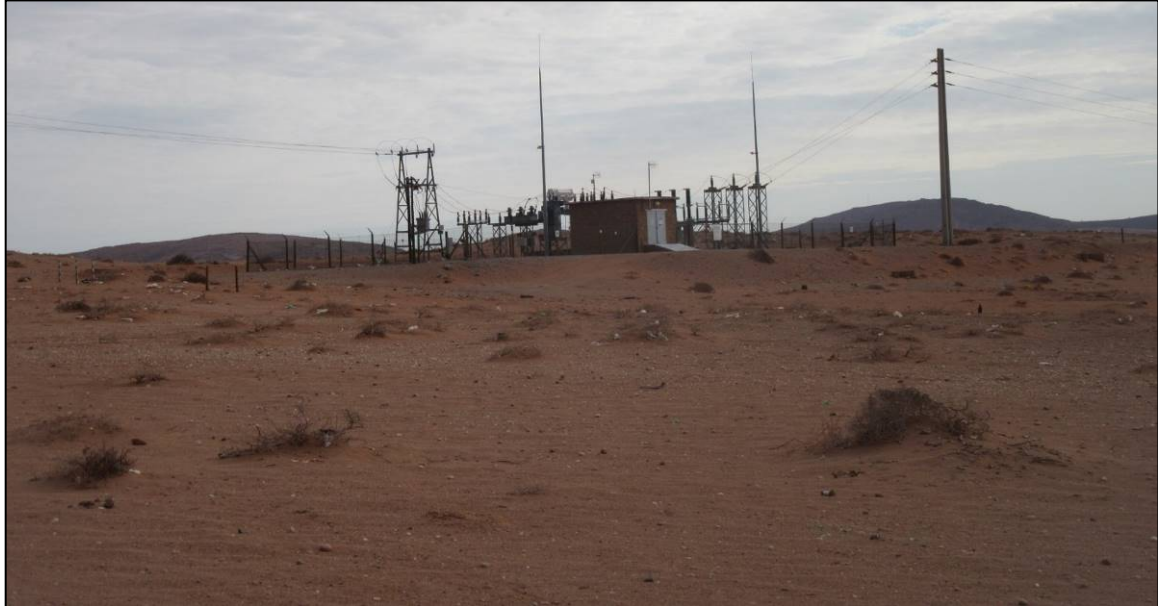
Photograph 3.6: The small Eskom substation on the western outskirts of Komaggas
