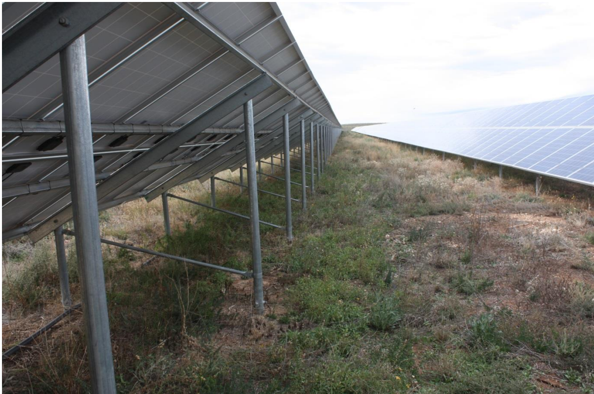
Figure 13: Image of solar arrays indicating the limited Influence that such structures generally have on the flow of surface waters within a solar facility.
