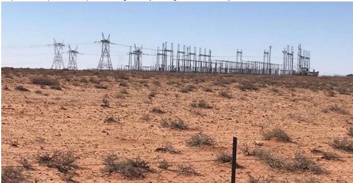
Figure 5: The 1 Aries – Nieuwehoop 400kV line where it terminates in the Nieuwehoop Substation.
