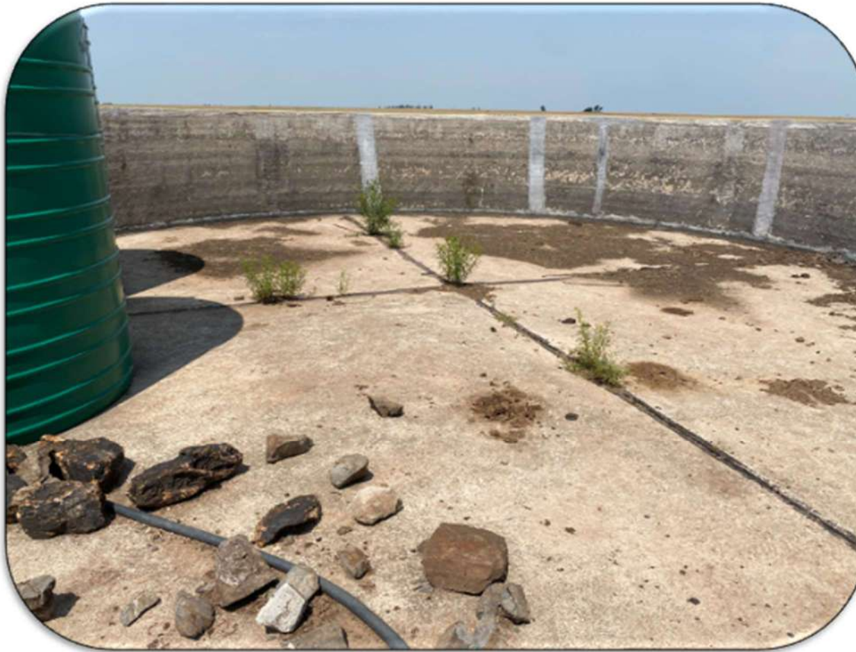
Figure 26: Photograph of the large broken cement reservoir located within the study area
