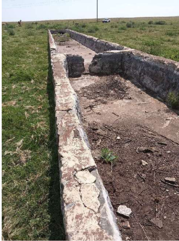
Figure 37: Close-up view of interior of the trough showing plaster and paint
