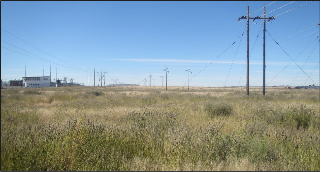
Figure 12: Looking east through the northern part of the powerline corridor from the R48. An existing SEF is visible to the left.
