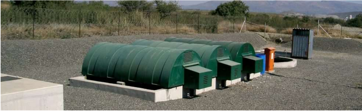
Figure 2: Typical example of WWTW
