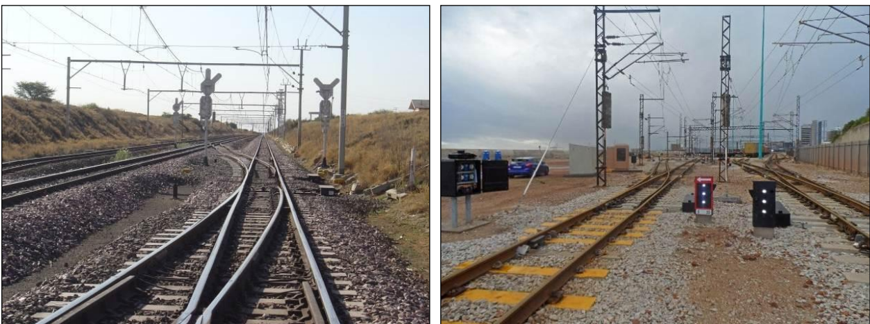
Figure 3.4: An example of a railway perway (left) and typical railway signalling (right).
