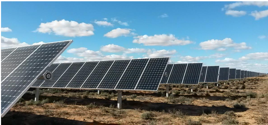
Figure 1: Solar Panels (Image: Mulilo Prieska PV)
