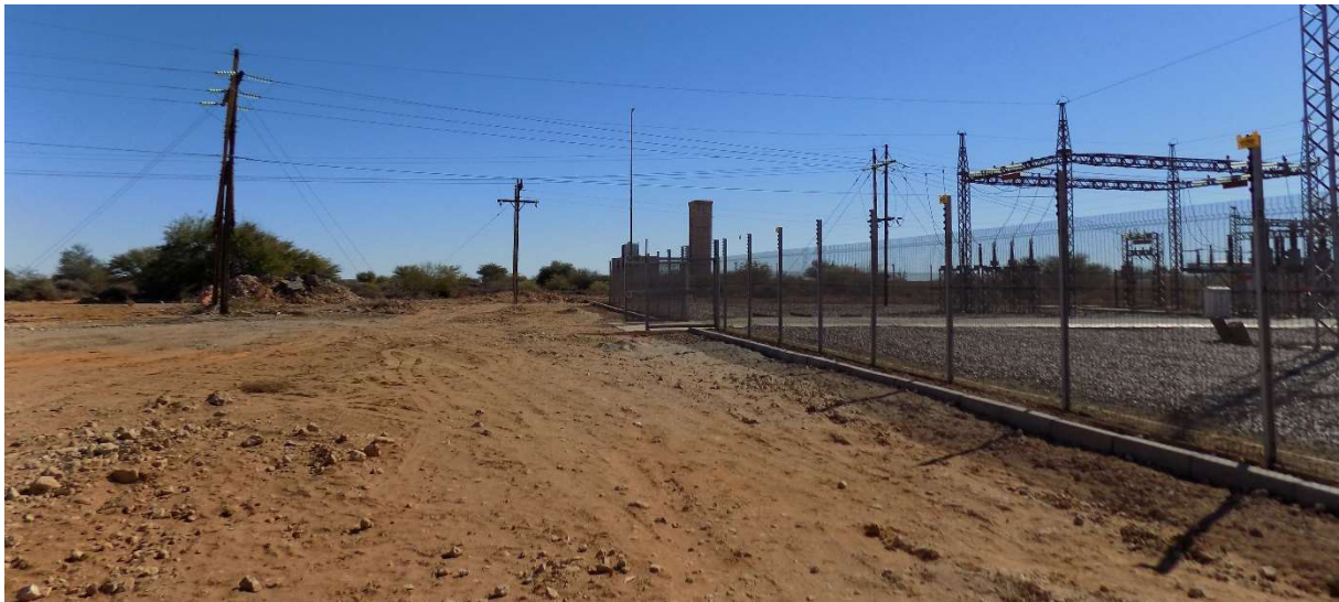
Photo 1: The Cuprum Substation with area proposed for extension in the foreground
