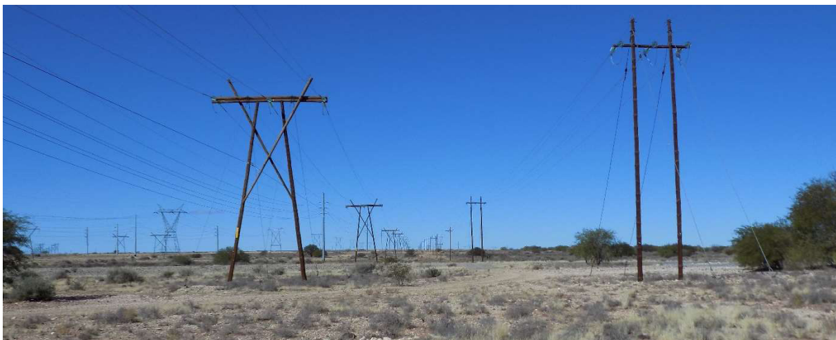
Photo 6: Example of bird friendly pole structures for 66kV (left) and non-bird friendly pole structures for 11kV (right)
