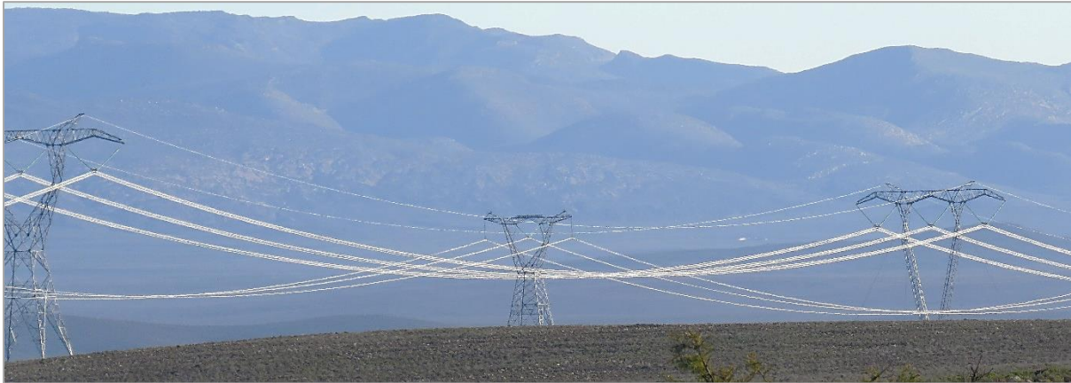
Photo 1: Example of staggered pylons, in which the tower of one OHPL is aligned with the mid-span of the adjacent OHPL in the Karoo. Theoretically, this should decrease the collision frequency of species such as bustards by 67%.
