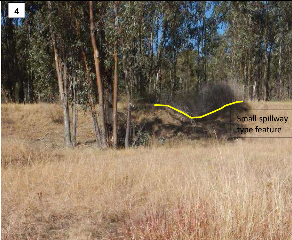
South eastern upstream view of small spillway type feature along the earth dam wall. Co-ordinates: 26°22'46.71"S; 27°57'55.82"E
