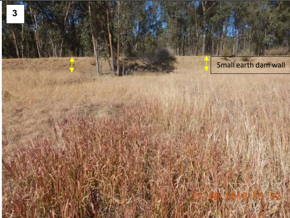
South eastern upstream view of the non-perennial river and small earth dam wall. Co-ordinates: 26°22'46.72"S; 27°57'55.82"E
