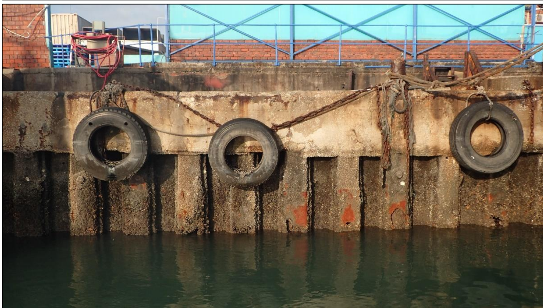
Figure 3. Photographs of part of the existing Old Tug Jetty sheet pile quay wall in the Port of Port Elizabeth. Note the damage to the sheet pile and concrete super structure.
