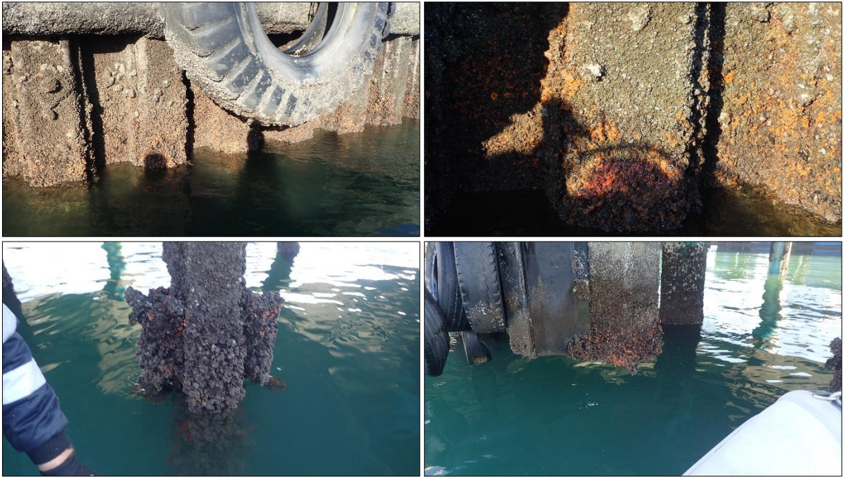
Figure 42. Photos showing encrusting organisms on the sheet pile quay wall at the Old Tug Jetty (top) and on piles near the Old Tug Jetty (bottom).
