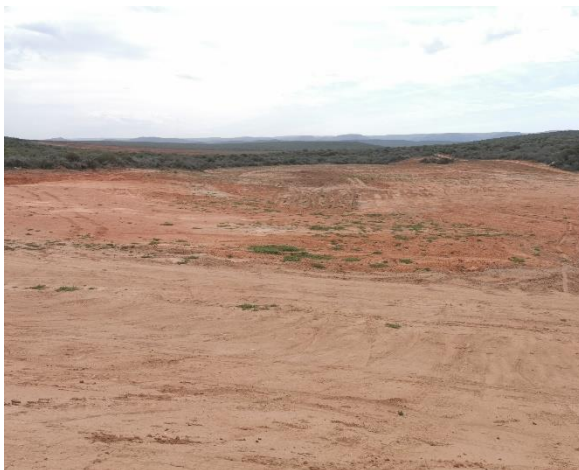
Figure 12: Clearance of vegetation on site for the smaller Scheepersvlakte Dam and expansion of citrus farming
