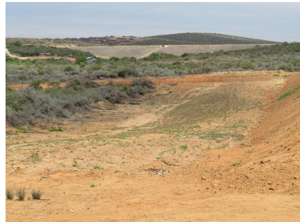
Figure 11: Smaller Scheepersvlakte Dam under construction immediately south of the proposed dam site
