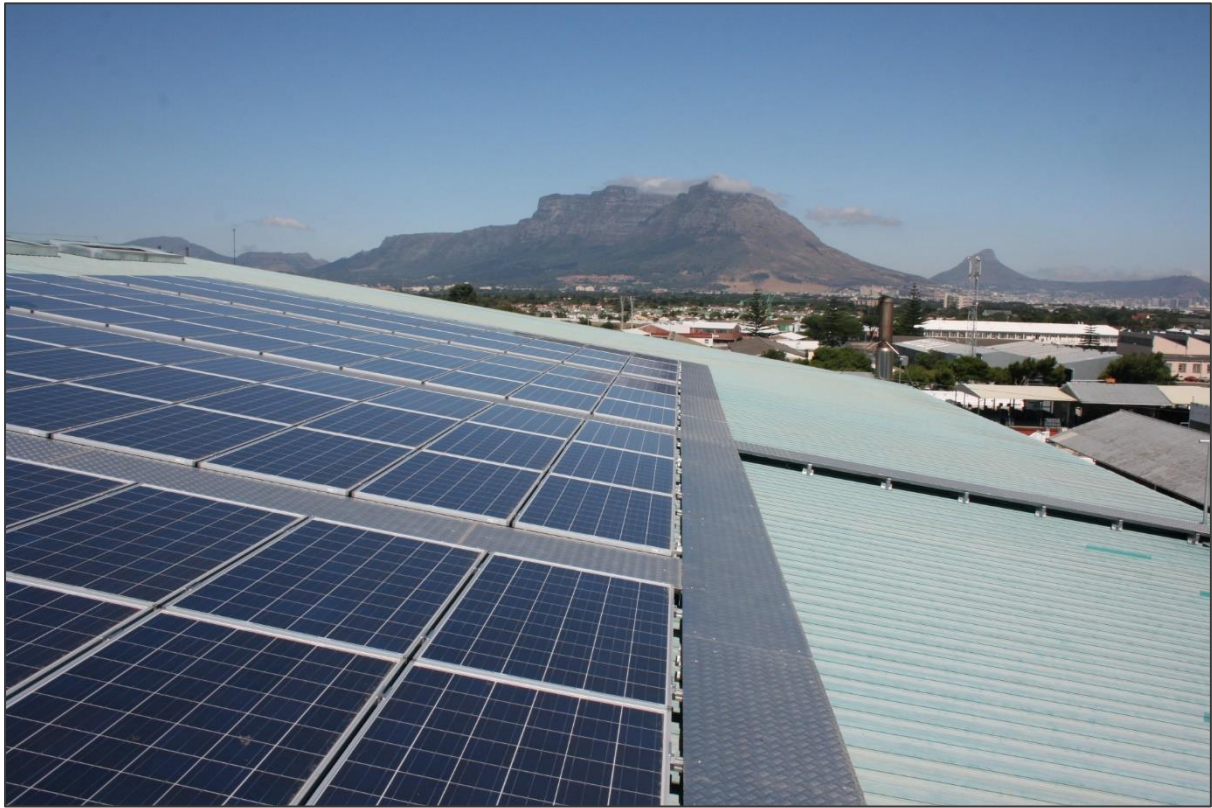
Figure 4.3: Solar Installations at the George Airport in the Western Cape
