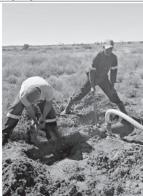
The Emthanjeni Municipality water works team busy with repairs on the Burgerville Main Line.
