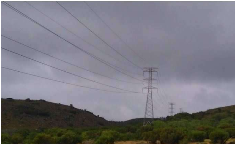
Figure 5: Example of a 132 kV transmission line
