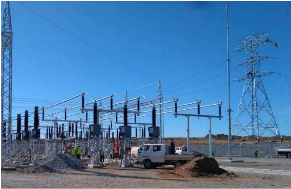
Figure 6: Example of High Voltage Transmission Line Connecting to Substation
