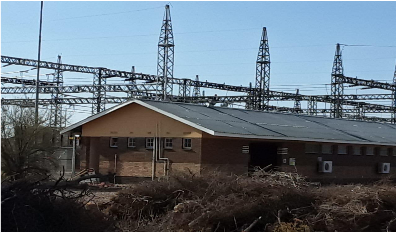
Plate 1: Photo 1: View of Cuprum Substation and related infrastructure (Photograph © by Author 2021).
