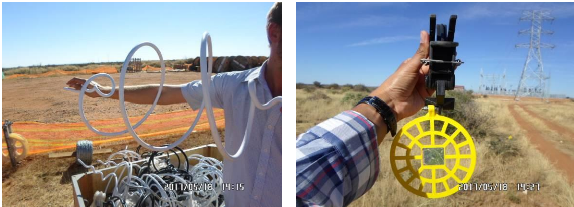
Figure 24: Examples of bird flight diverters to be used on the power lines: Double loop bird flight diverter (left) and Viper live bird flapper (right).
