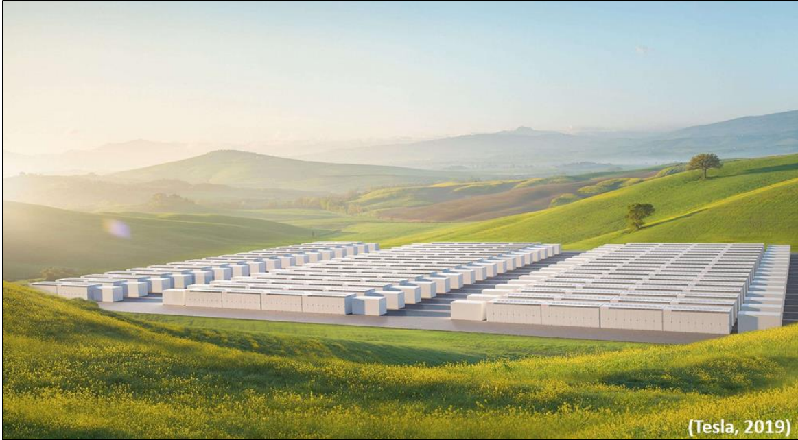
Figure 1: Tesla's Megapack Li-ion Battery (Modular System).
