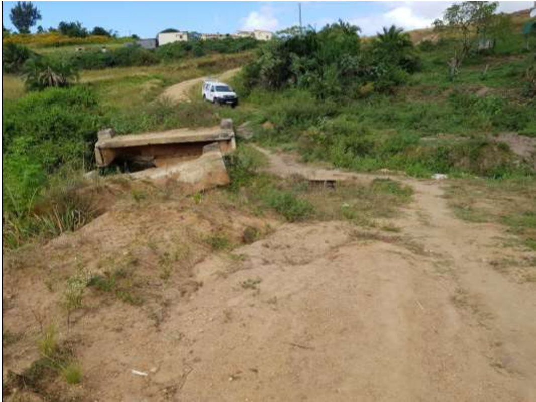
Plate 3: General view across the site viewing in a southerly direction. Note collapsed bridge.
