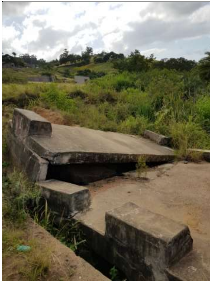
Plate 4: General view of collapsed concrete river bridge
