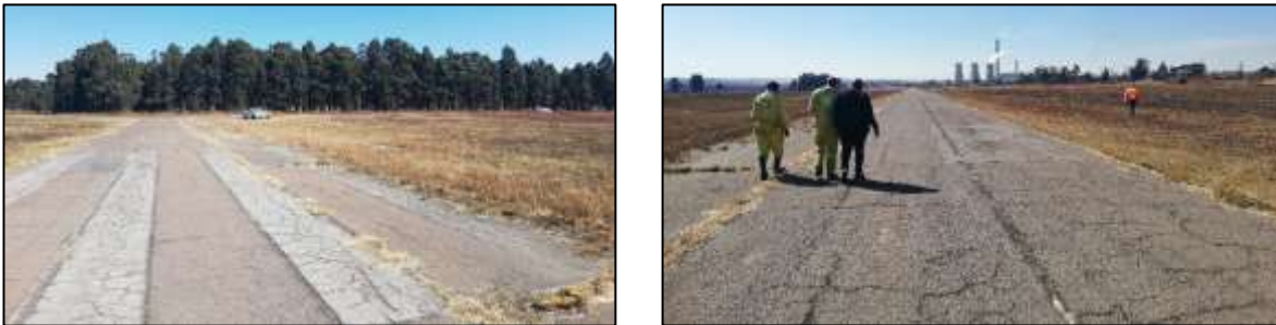
Figure 1: Condition of the airstrip at Koorfontein Mines
