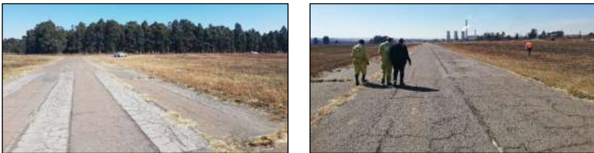
Figure 1: Condition of the airstrip at Koorfontein Mines
