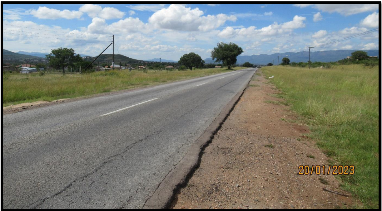
Figure 10: View of road with wide shoulder, lush grass and deteriorating surface.
