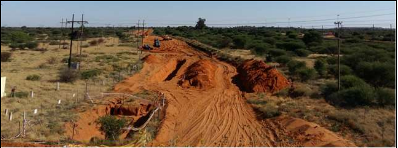
Figure 7: To the west of the railway line, large sections of the landscape on the Remaining Extent of farm York A 279 have been disturbed by the construction of an underground water pipeline which runs parallel to the railway line, and between the railway line and the R31. Note also the 66kV powerline which crosses the site from east to west.
