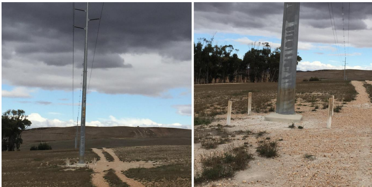
Plate 7: Example of the extent of the disturbance footprint of a 132 kV pylon (Photo: J Gribble, Excelsior WEF grid connection).
