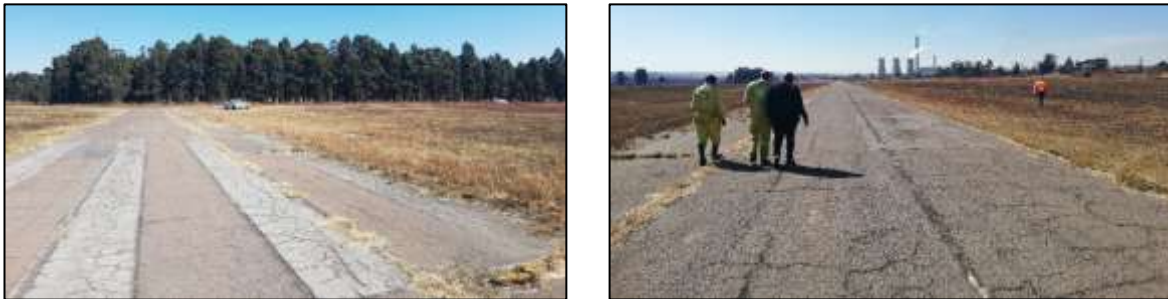
Figure 1: Condition of the airstrip at Koorfontein Mines
