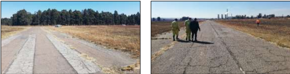
Figure 1: Condition of the airstrip at Koorfontein Mines
