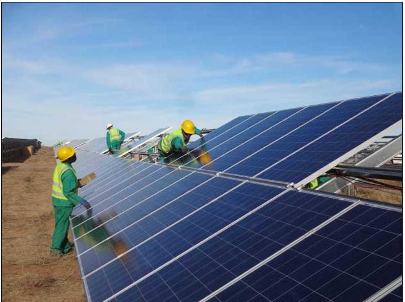
Figure 4: Solar panel arrays ( http://www.popularmechanics.co.za )
