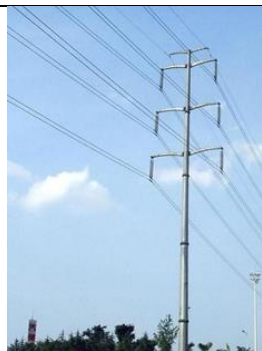
Plate 6-1: Concrete, steel or wood monopoles.
