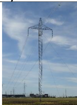
Plate 6-3: Free standing metal lattice towers.
