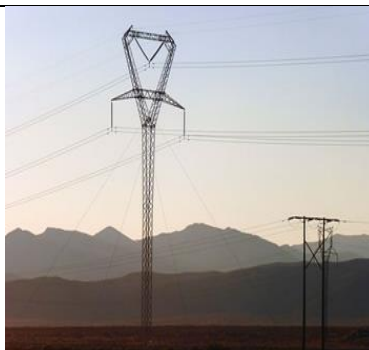
Plate 6-2: Guy line supported steel structures.
