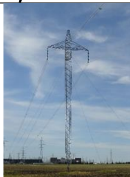
Plate 6-3: Free standing metal lattice towers.
