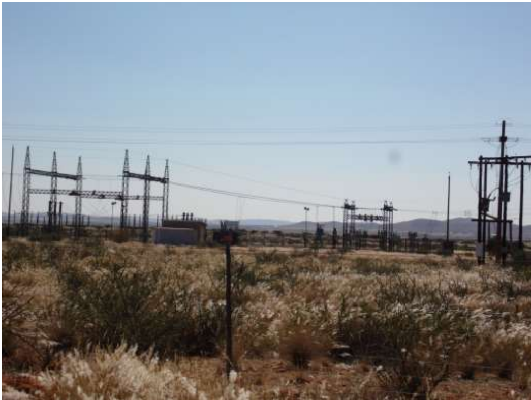
Figure 22 | Eskom’s Fibre substation where the transmission line would connect to the national grid
