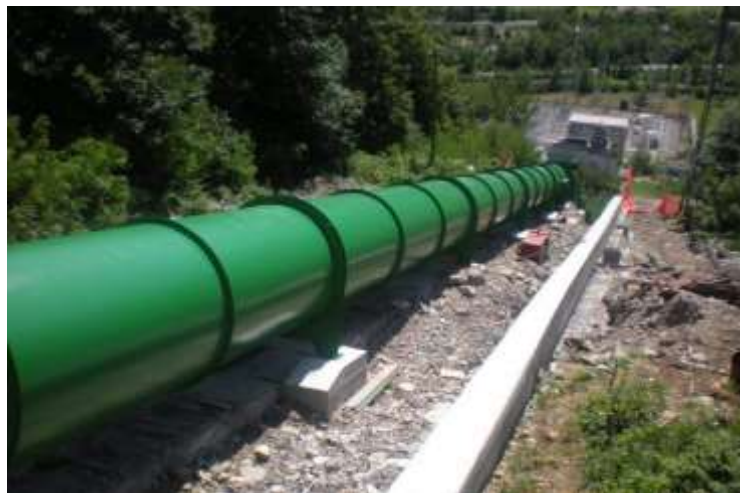
Figure 16 | Example of a penstock (source: energypedia.info (Accessed: 28 June 2013)).
