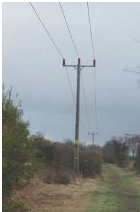
Figure 21 | Example of a 33kV transmission line (Source: www.electrical-contractor.net (Accessed 9 September 2013))
