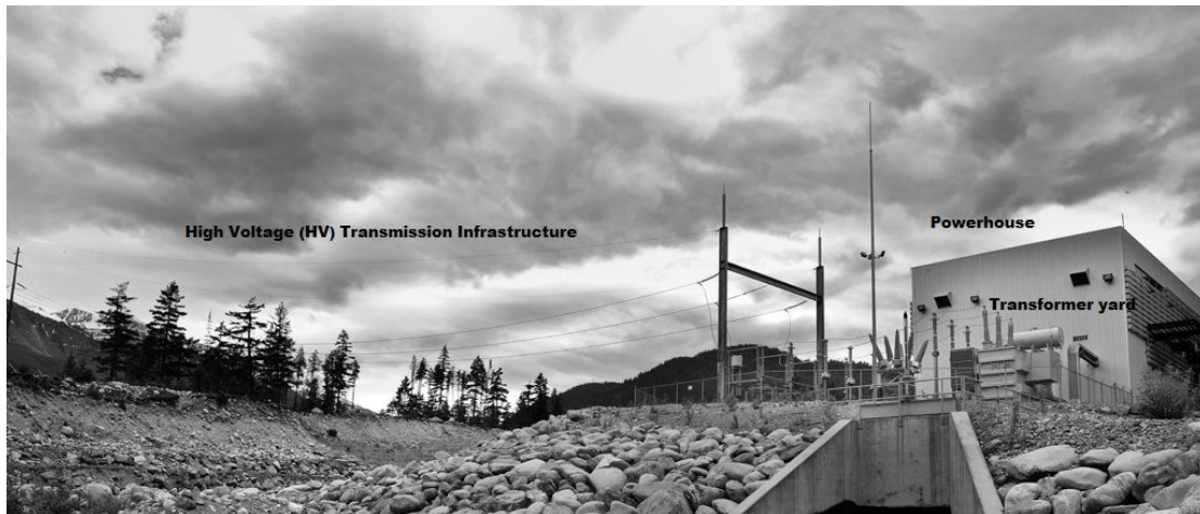
Figure 19 | Example of a power chamber and associated infrastructure (source: http://www.photosensitive.com (Accessed: 28 June 2013))
