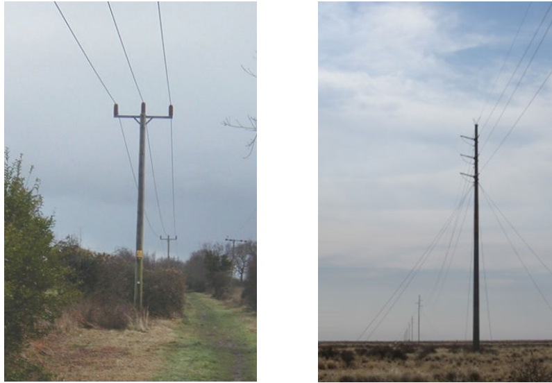
Figure 20 | Example of a 33kV transmission line on the left and a 132kV transmission lines on right (Source: www.electrical-contractor.net (Accessed 9 September 2013))
