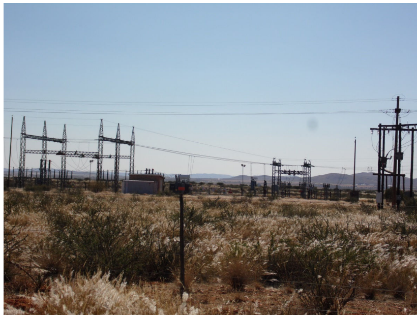
Figure 21 | Eskom's Fibre substation where the transmission line would connect to the national grid
