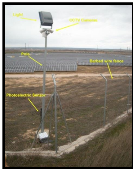
Figure 11: Example of security system elements
