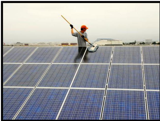
Figure 13: Cleaning PV panels
