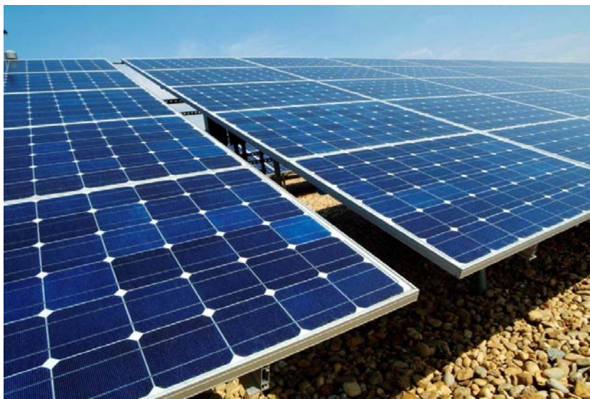
Figure 2.2: Photograph illustrating photovoltaic panels
