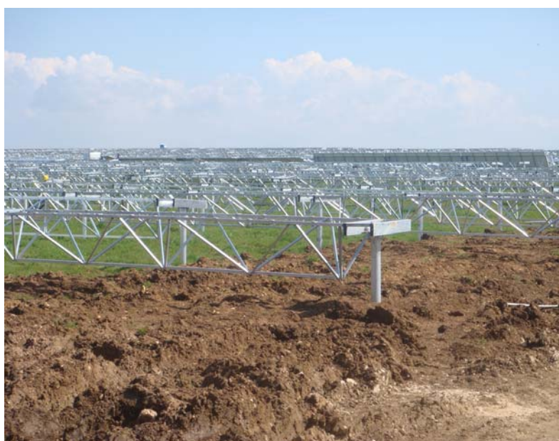
Figure 2.4: An example of site preparation activities that required the levelling some sections of the site.
