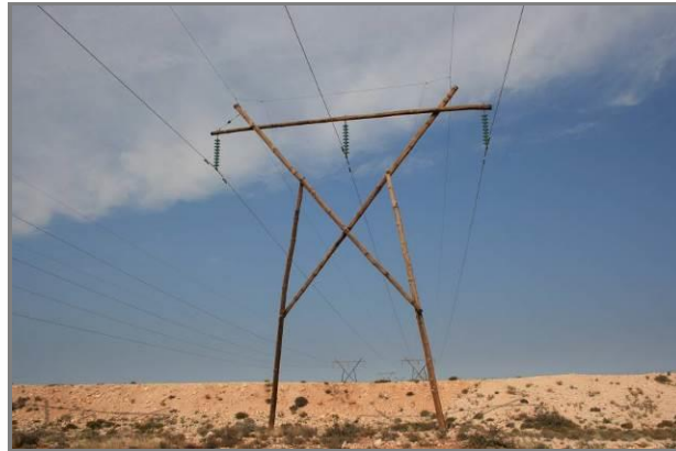
Figure 2.4 Example of an existing 132 kV transmission line (taken 29/09/2011)
