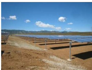
Fig 2.3: Image of Ray tracker utility scale solar tracker installation, tech. Option 1. Source Mulilo
