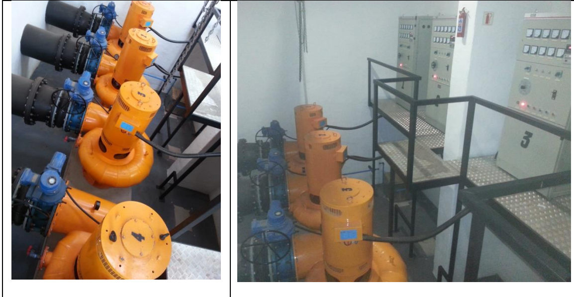
Figure 1: Examples of the turbines (spiral casings in orange) in a parallel manifold with generators (on top of the spiral casings, also orange) and turbine system controllers (grey boxes) inside the hydro power house
