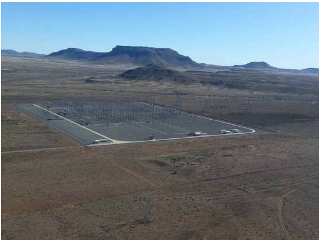
A view of the existing Gamma Substation.
