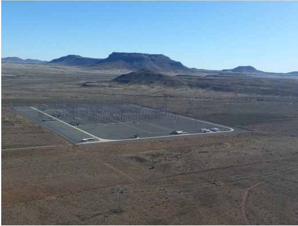
Plate 5: The Gamma Substation and a powerline in the foreground in a flat open plan, with koppies and mesas in the background.
