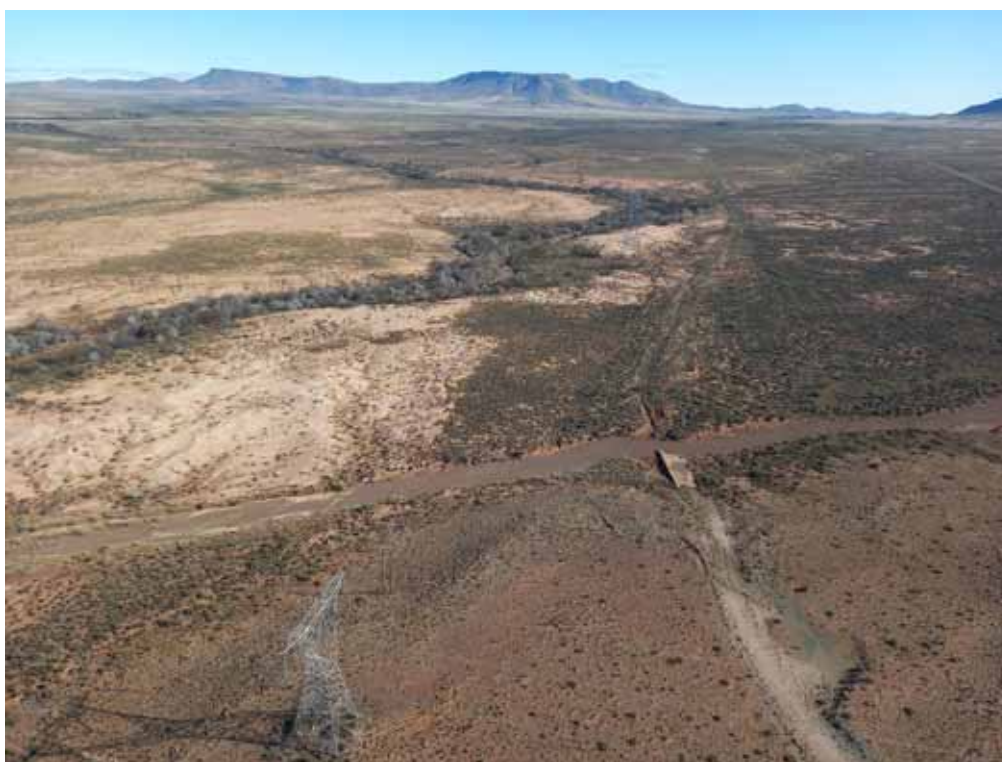
Plate 8: An existing track over a drainage line that has been washed away. High rainfall occurred just prior to the photograph being taken (i.e. July 2022). Access roads over drainage lines need careful placement and design.
