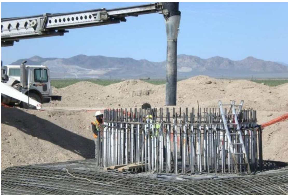
Figure 5.1: Photograph illustrating the construction of the foundation for a wind turbine (photo sourced from www.blm.gov )
