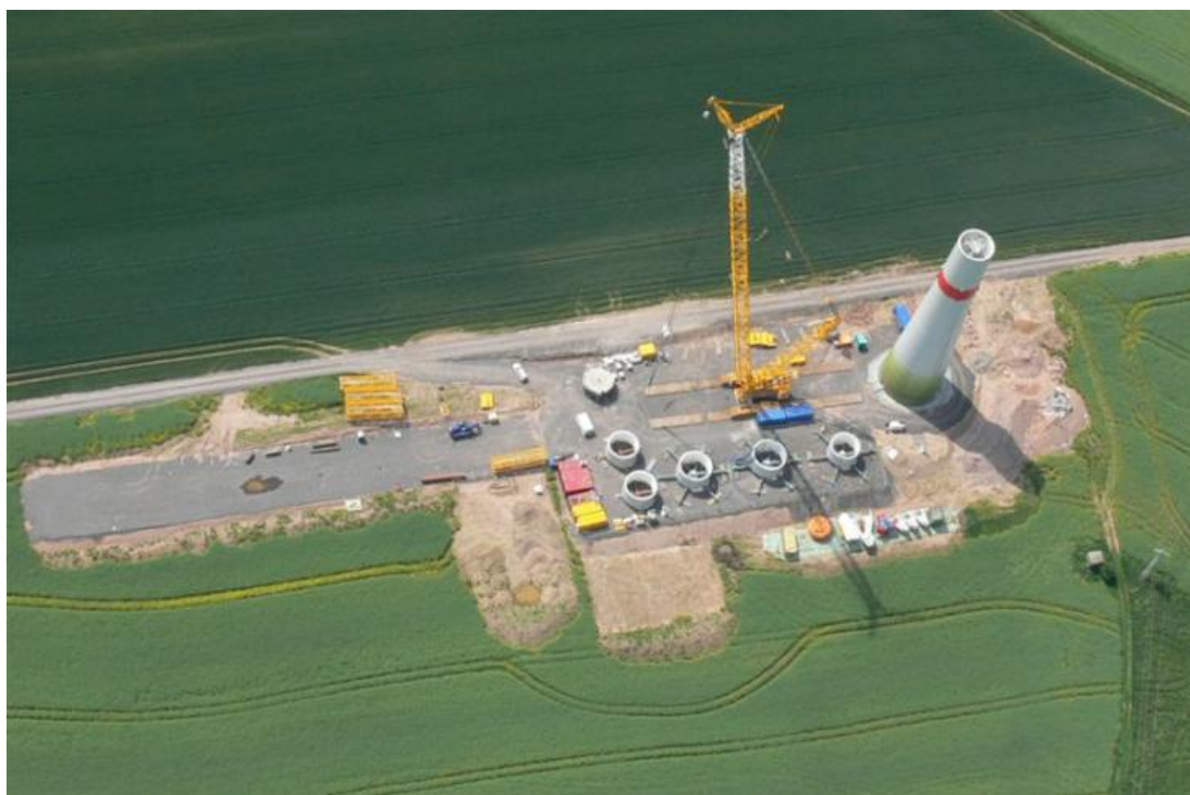
Figure 5.3: Photograph illustrating an example of laydown areas for a wind turbine. The soil stock piles to be reused during rehabilitation can also be seen around the laydown area (photo sourced from www.juwi.com )
