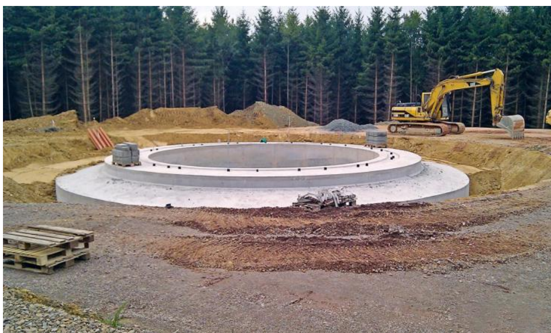
Figure 5.2: Photograph illustrating a completed foundation for a wind turbine (photo sourced from www.juwi.com )
