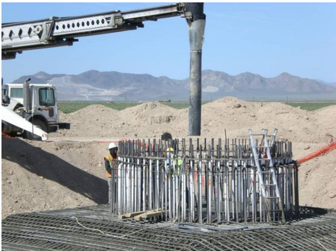
Figure 7.2: Photograph illustrating the construction of the foundation for a wind turbine (photo sourced from www.blm.gov )
