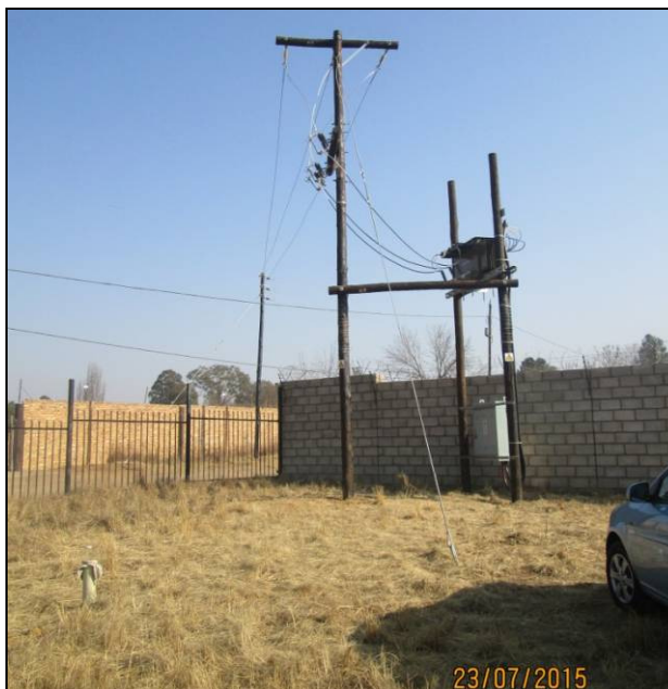
Photo 3.7: A view of the Eskom Transformer and power lines
