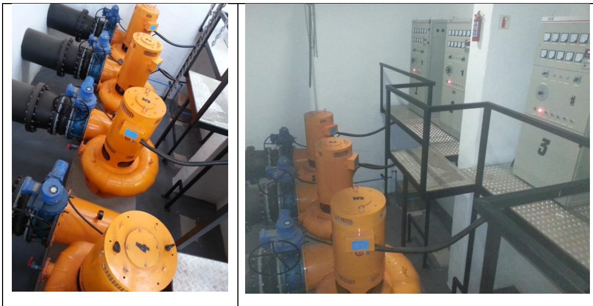
Figure 1: Examples of the turbines (spiral casings in orange) in a parallel manifold with generators (on top of the spiral casings, also orange) and turbine system controllers (grey boxes) inside the hydro power house
