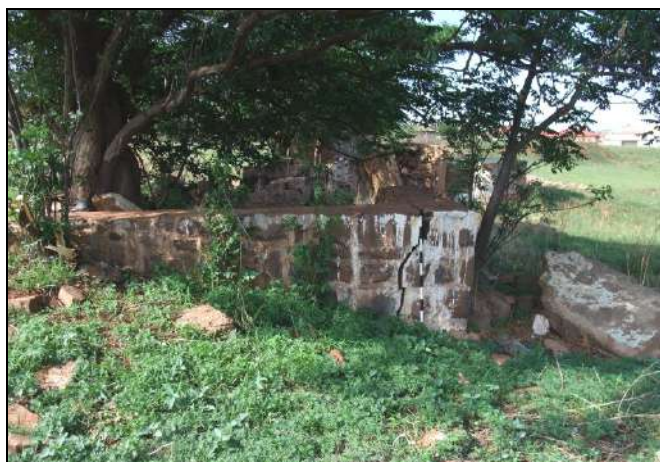
Photo 5.16: Remaining stone wall that may have been the foundation of a farm house
