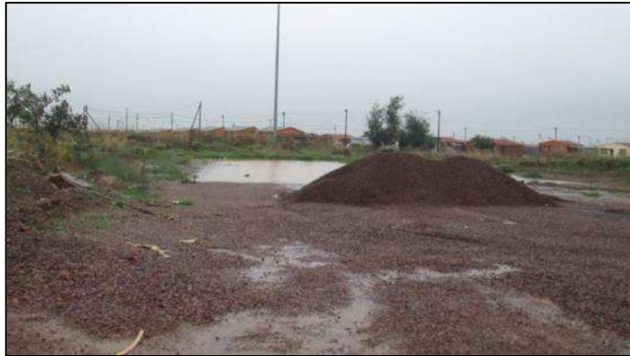
Photo 5.14: Ponding within the construction material storage area
