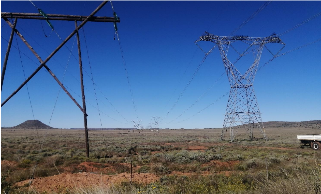
Figure 5.21: Electrical infrastructure that traverses the study area
