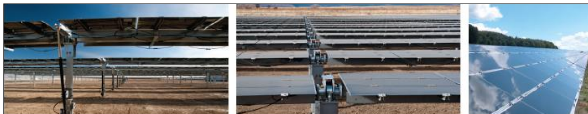
Figure 3: Examples of Solar PV Tracking System (Source: First Solar)
