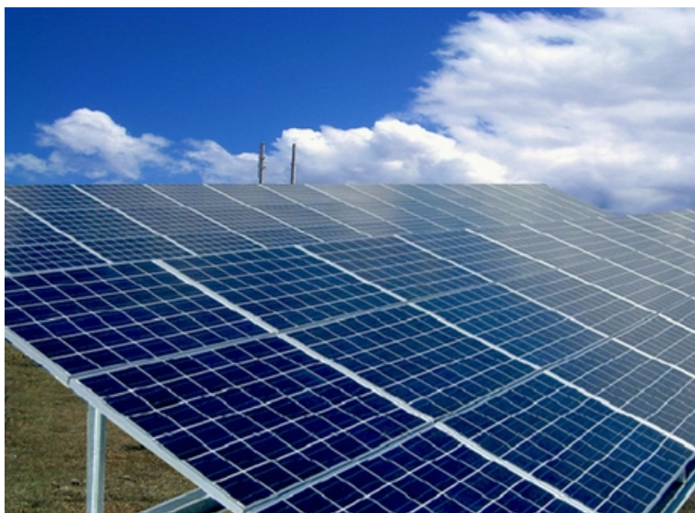
Figure 2.2: Photo showing view of photovoltaic panels.
