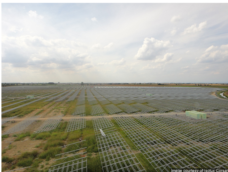
Figure 2.5: Example of erected steel mounting structures awaiting the installation of the PV panels (SunEdison Photovoltaic Power Plant, Rovigo, Italy)
