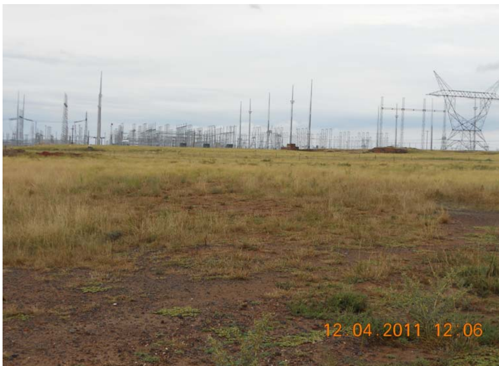
Figure 5.1: A distant view of Hydra Substation and surrounding power lines
