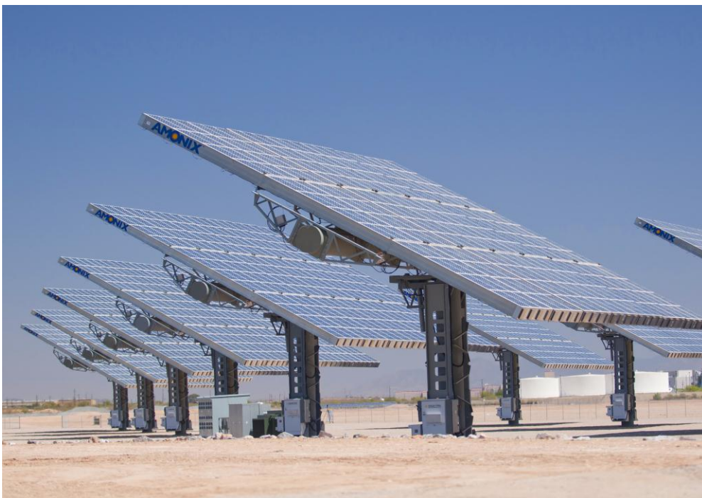
Figure 4: The support structures elevate the panels by 15 m and allow for dual axis tracking of the sun for increased efficiency (Courtesy of Amonix™)
